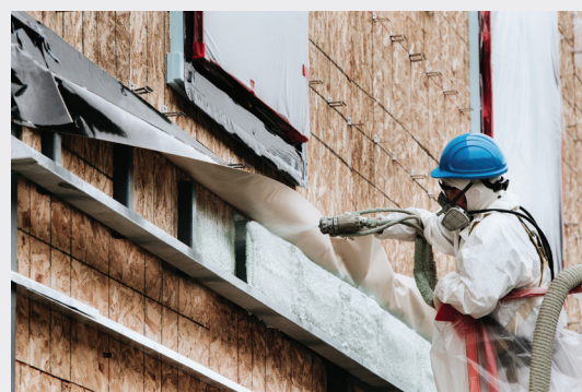
Figure 3: Installation of polyurethane spray foam to a wall (photo courtesy of Huntsman International LLC).
