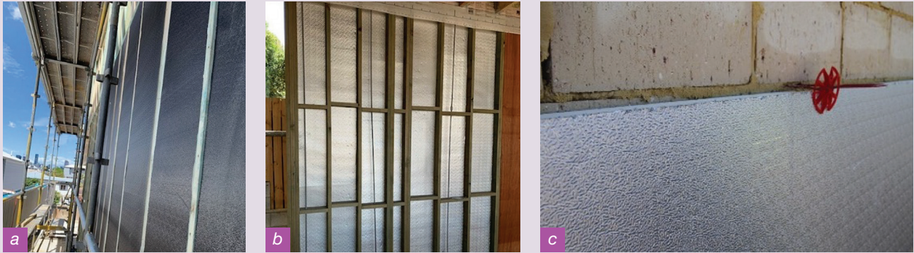
Figure 1: a) and b) Foil faced PIR insulation board installed external to the frame (continuous insulation) on a low-energy house in Brisbane prior to installing cladding (photos courtesy of Pirmax Pty Ltd), c) Foil faced PIR insulation board being installed in the cavity of a double brick construction (photo courtesy of Reflex Insulation Pty Ltd).
