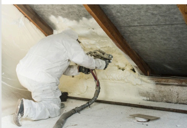
Pacific Urethanes Spray Foam insulation
